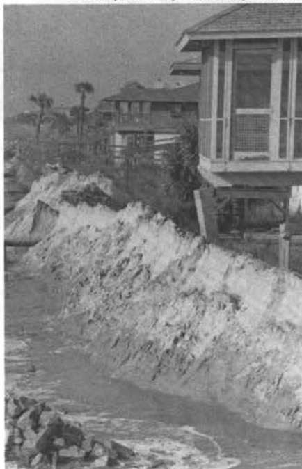
WINTER STORMS BATTER THE REVETMENT ON FRIPP ISLAND.
