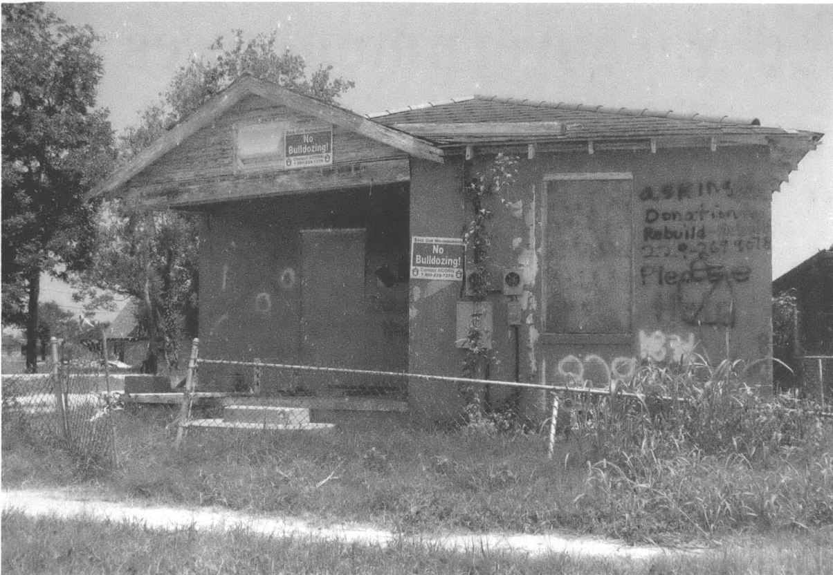
Lower Ninth Ward, August 2007. Shortfalls, delays and mismanagement of federal programs have kept money from flowing to home rebuilding and other Gulf Coast recovery efforts.
