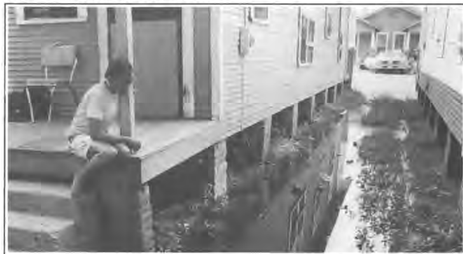
STAGNANT WATER FROM A BROKEN TOILET DRAINPIPE IS A CONSTANT COMPANION FOR BANKS STREET RESIDENT PATRICIA STOKES.
