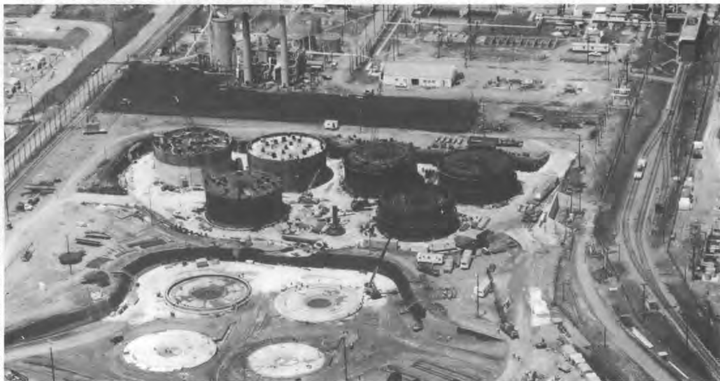
AERIAL PHOTO OF WASTE TANKS UNDER CONSTRUCTION AT THE SAVANNAH RIVER PLANT. BACKGROUND SHOWS CHEMICAL SEPARATION FACILITIES WHERE IRRADIATED FUEL IS REPROCESSED.
