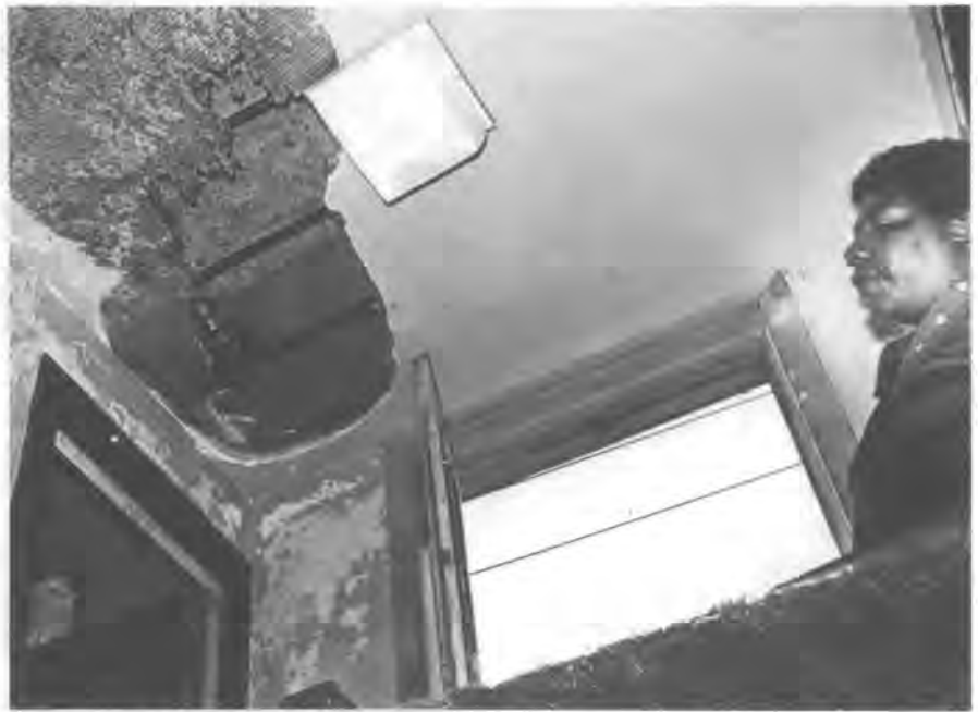
FALLING CEILINGS ARE A MAJOR HAZARD IN THE ST. THOMAS HOUSING PROJECT.
