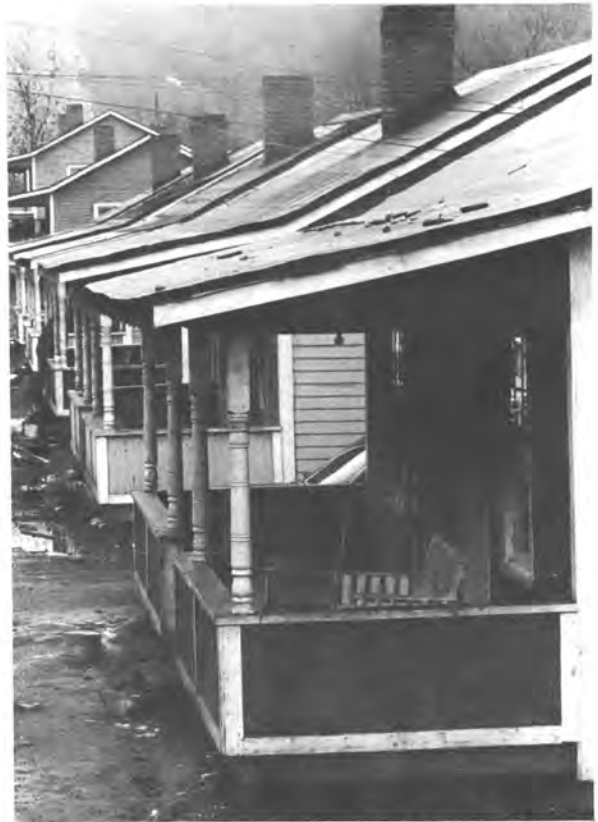
Houses in the Brookside camp still lack indoor plumbing; consequently, raw sewage from out-houses pours directly into the nearby stream.
